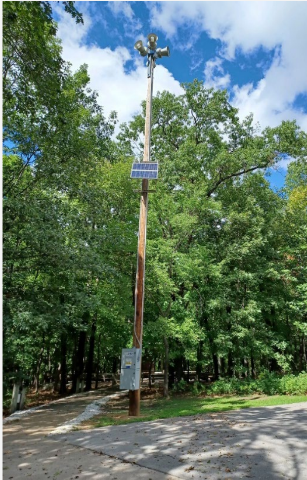
Example siren installed at Mark Twain State Park
